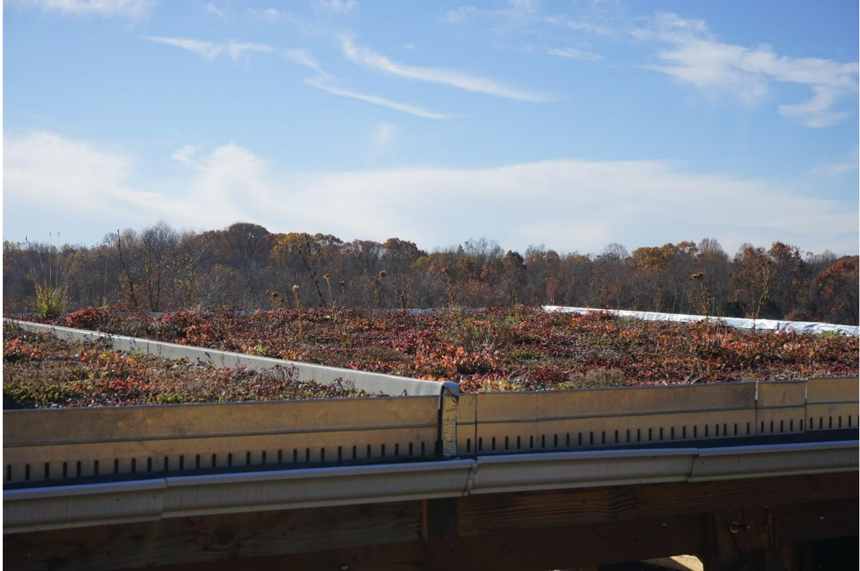
Figure 23. Two Extensive Green Roof Demonstration at Knoll Farm
